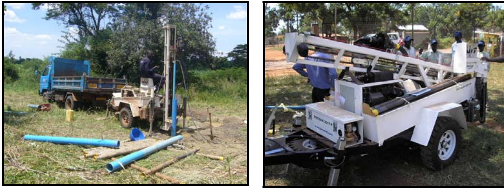
Figure 4: The TGS Water PAT301 TP rig
